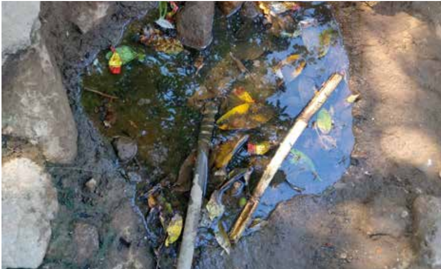
Broken water stand pipe at Kaleyia Smallholders
